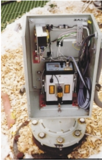
LD90-450 installed in a flange mount enclosure
