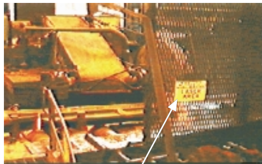
Laser warning signs @ south east corner of 5 saw.
