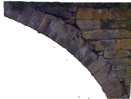
Figure 8. Coloured scan of a crack in an arch ring of Traba Bridge.
